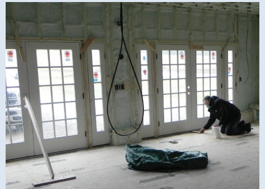
Fred Weston of Stillwater Sustainable Homes, LLC is overseeing the renovation of YLT's new community room.
